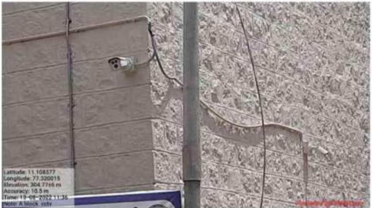
CCTV IN A BLOCK
