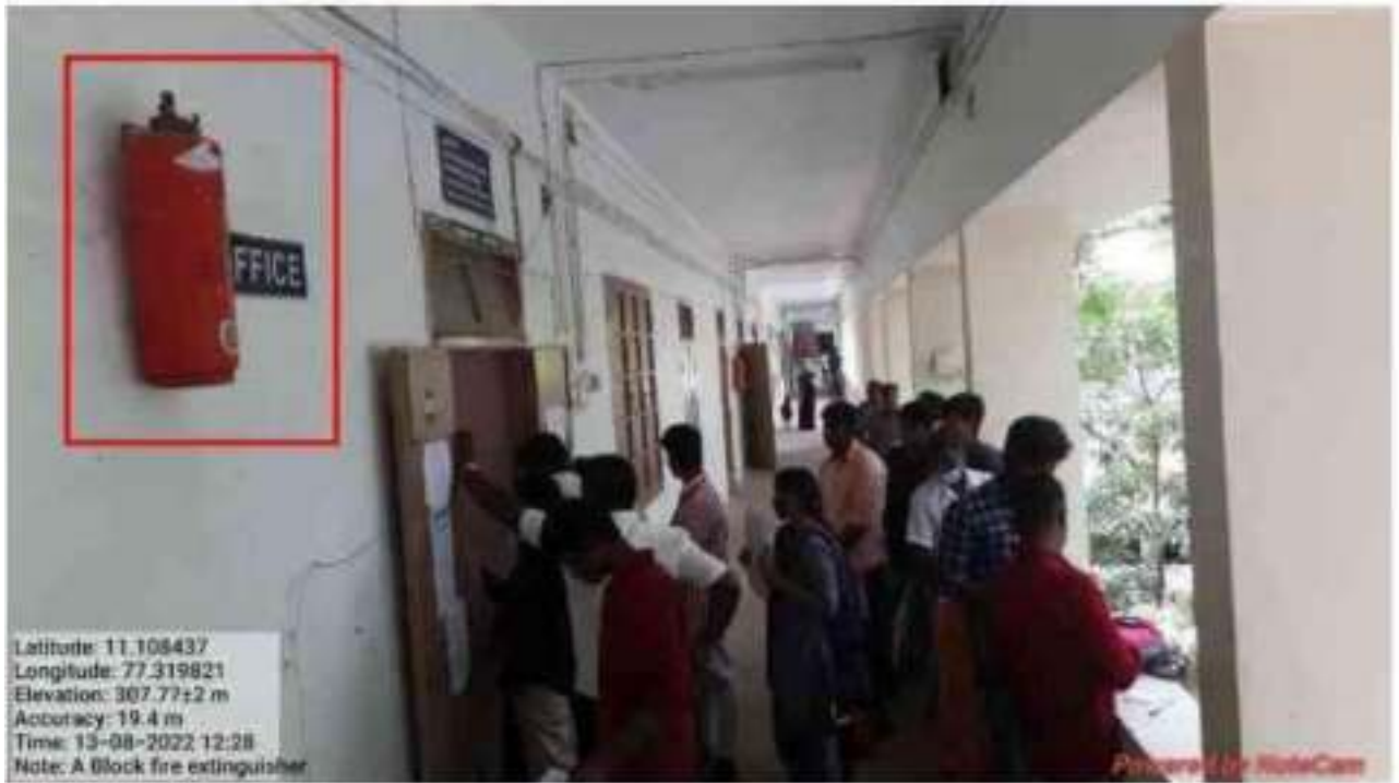
FIRE EXTINGUISHER IN A BLOCK
